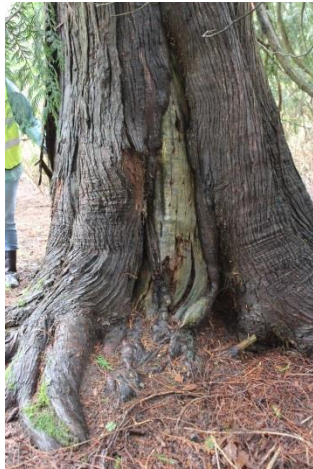
#1550 exposed roots with decay, large column of dead wood, carpenter ants and woodpecker
